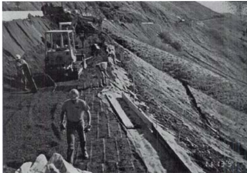
Figure 4. Wrapped face installation in conjunction with GSE embankment construction. 1:1.5 (H:V) Slope face gradient.
