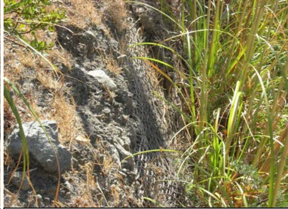
Figure 6B, View of twisted wire mesh and netting with vegetation
