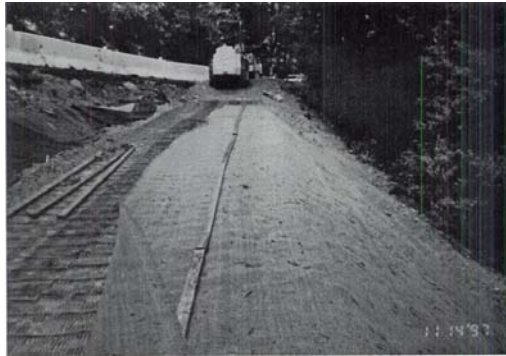
Figure 4A. Wrapped face construction abandoned due to wet grade. 1:1.5 (H:V) Slope face gradient.
