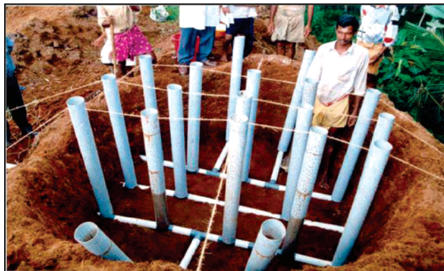
Figure 6. Initial assembly of the design of our composting assembly for coir pith.
